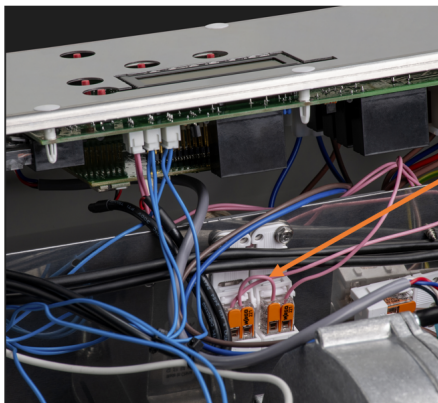
Looped Pink Wire – Fireman's switch connection
